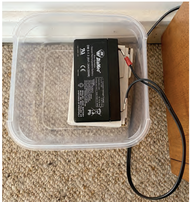
Figure 4-8 Battery location beside the clock
